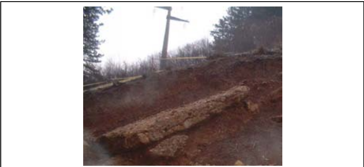
figure 66: The electricity cable closed to the measuring area. The high voltage influenced the 100 MHz radar measurement.
